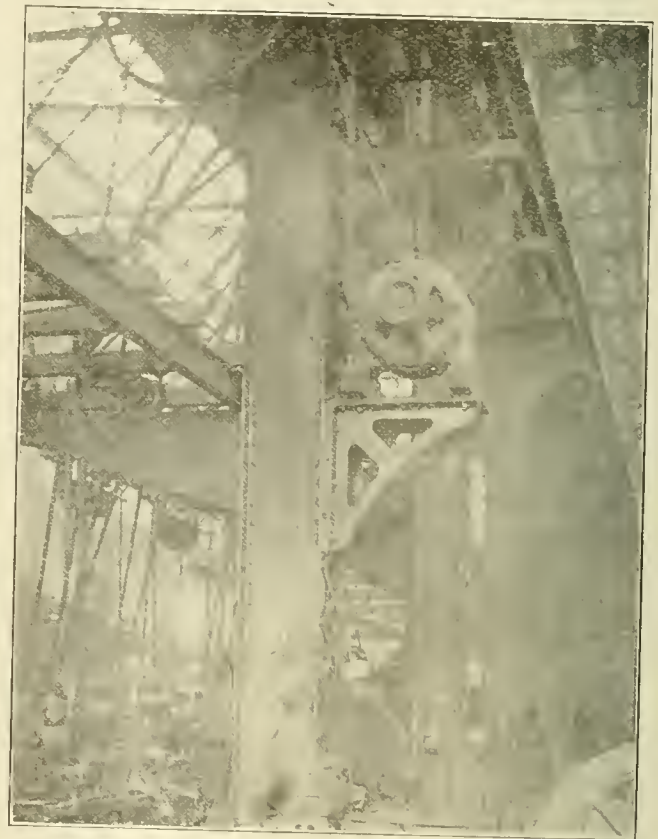
CLOSE VIEW OF MOTOR—SHOWING BRACKET SUPPORTS—EAST SIDE OF MACHINE SHOP BAY.
